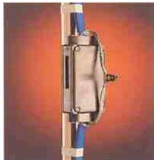
HEATING CABLE SPLICE
